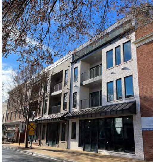
The Harris Building addition on Battle Street is in the final stages of construction.
