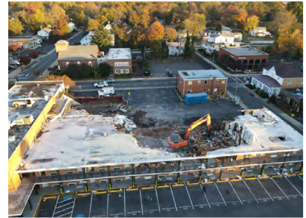
Demolition of the Olde Towne Inn is complete and redevelopment is coming.
