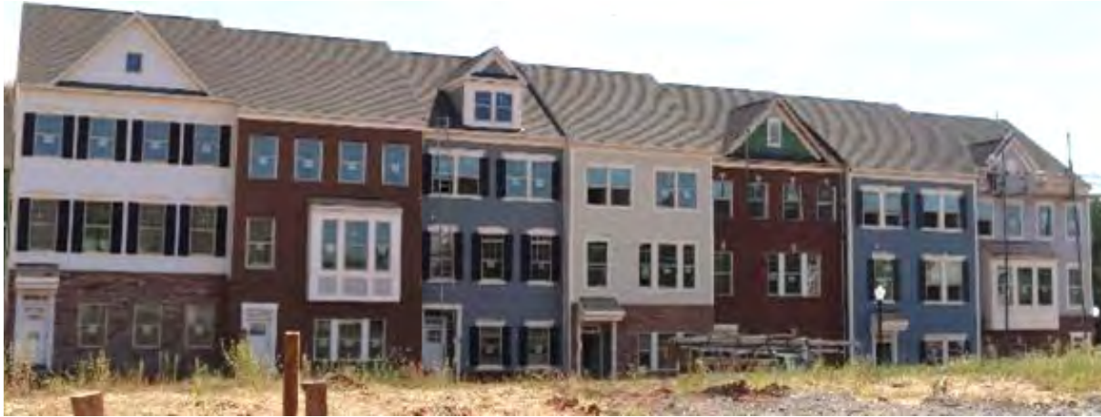
The Jefferson Square project at Prince William Street and Jefferson Street includes 85 townhomes and 20 single family homes. The project is nearing completion.
